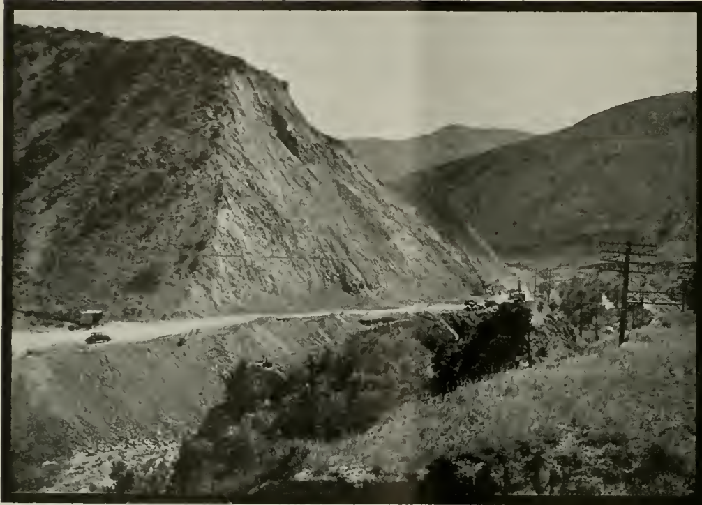
On the El Cajon Pass project, J. P. Holland, Inc., and Healy-Tibbitts Construction Company cut through the Blue Slide
